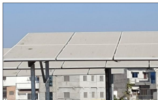
Figure 1 The accumulation of heavy amount of small dust particles onto a PV glass surface
