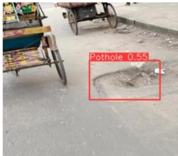
Figure 7 Sample Output of our Pothole Detection System by YoloV8 Model.
